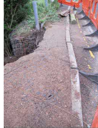
Gabion baskets installed before June 2009, disjointed kerbing, sloping metal posts of the safety barrier.
